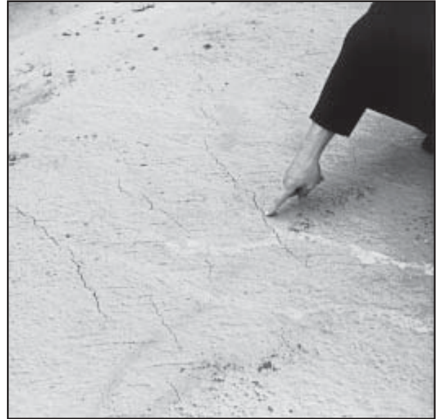
Plastic Shrinkage Cracks
