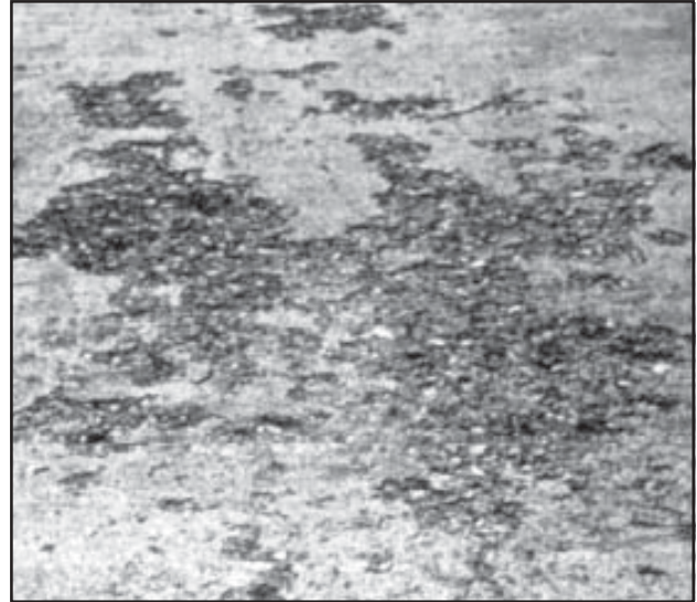
Scaling concrete surface
